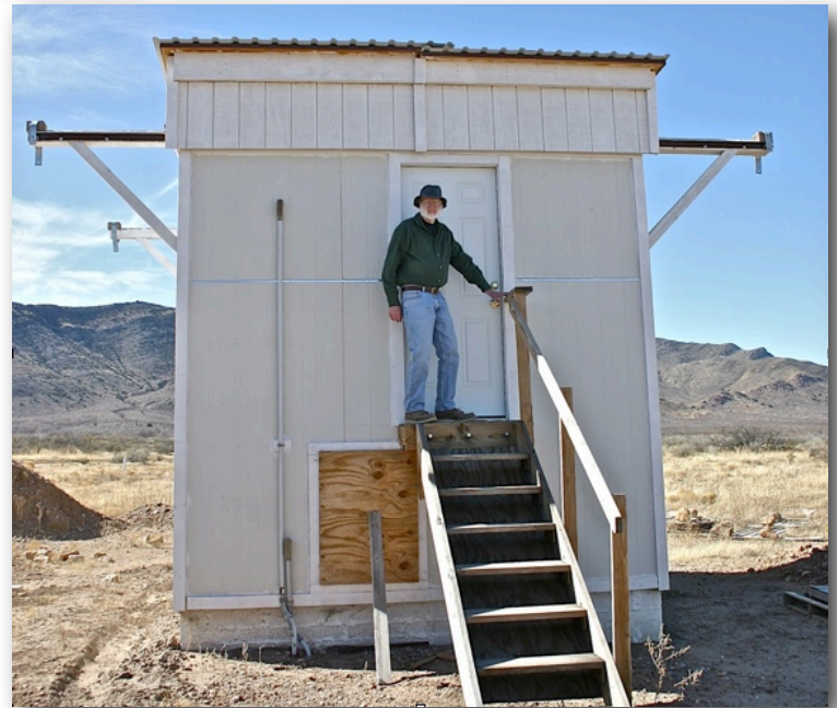
Jim Algots’ Split-Roof Research Observatory is almost finished
